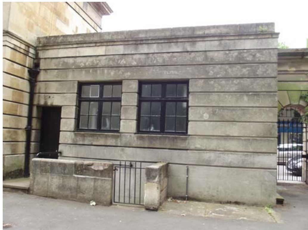
11. North Lodge - East Wing, south elevation showing mid 20th century cement render and altered windows and original door blocked up. Refer MRDA render removal study
